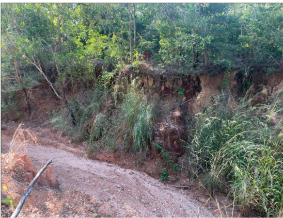
Figure 2-1 – Erosion Gullies Example 1
