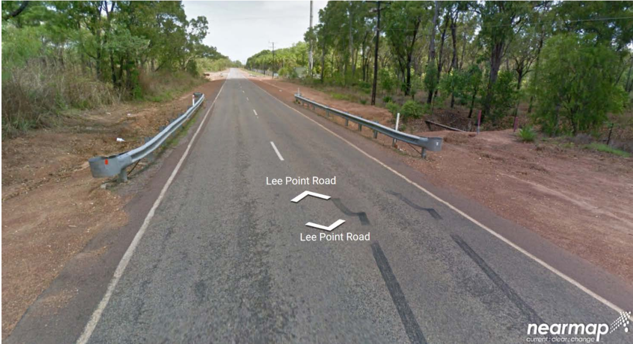
Figure 1-2 Culvert Crossing of Lee Point Road 115m South of the Lee Point Resort (Ref: Nearmap 2016)
