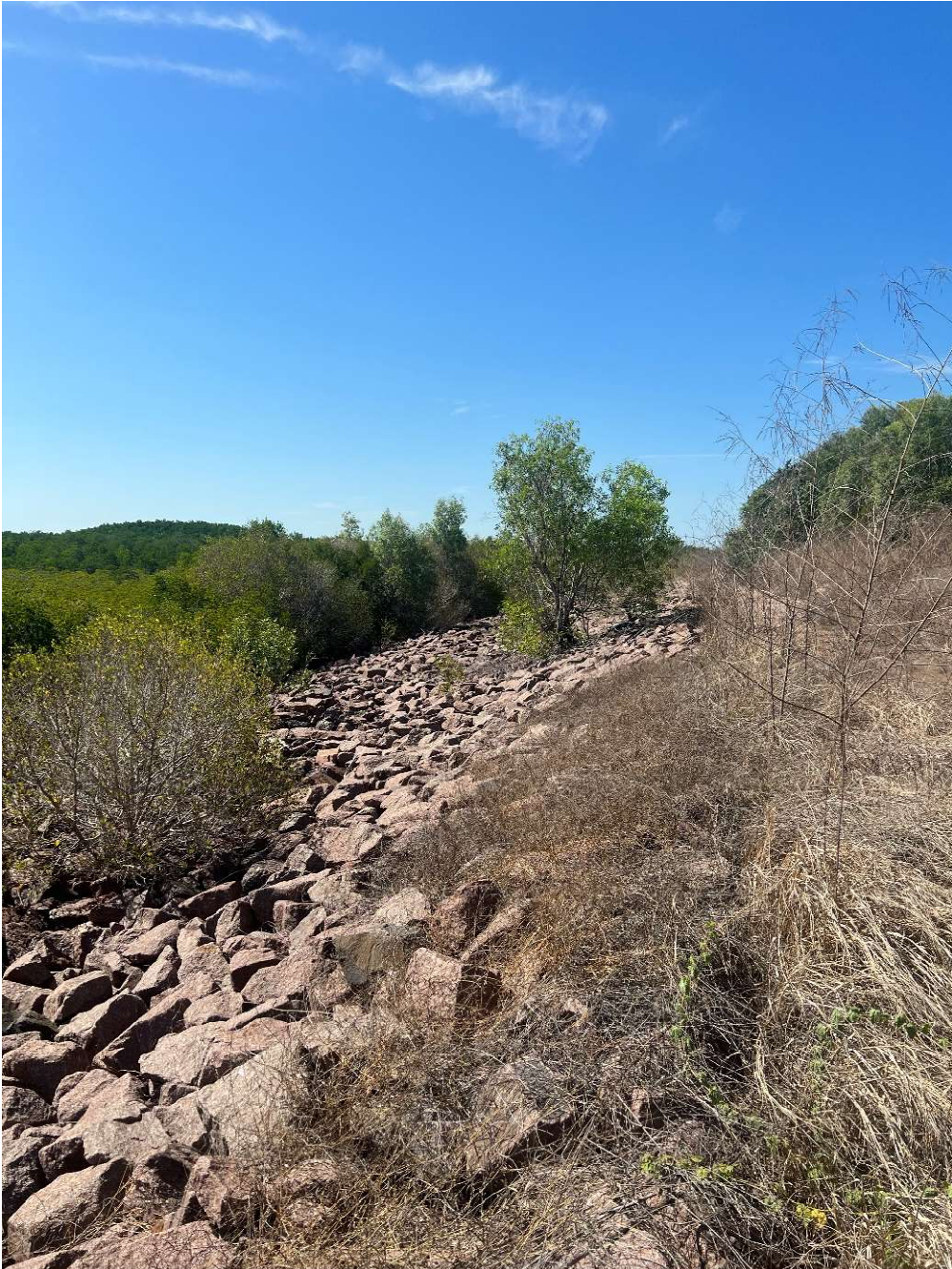
A view along part of the existing seawall on the eastern side of Bayview
